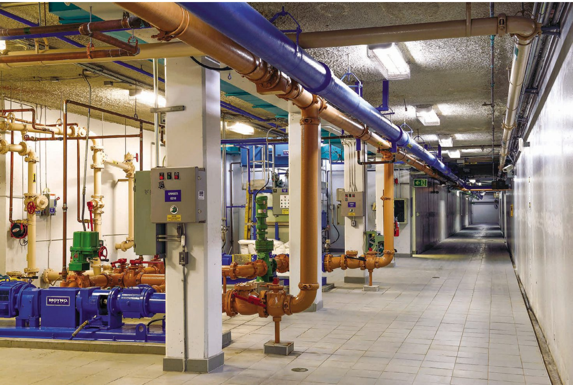
Inside the Riverview wastewater treatment facility.
