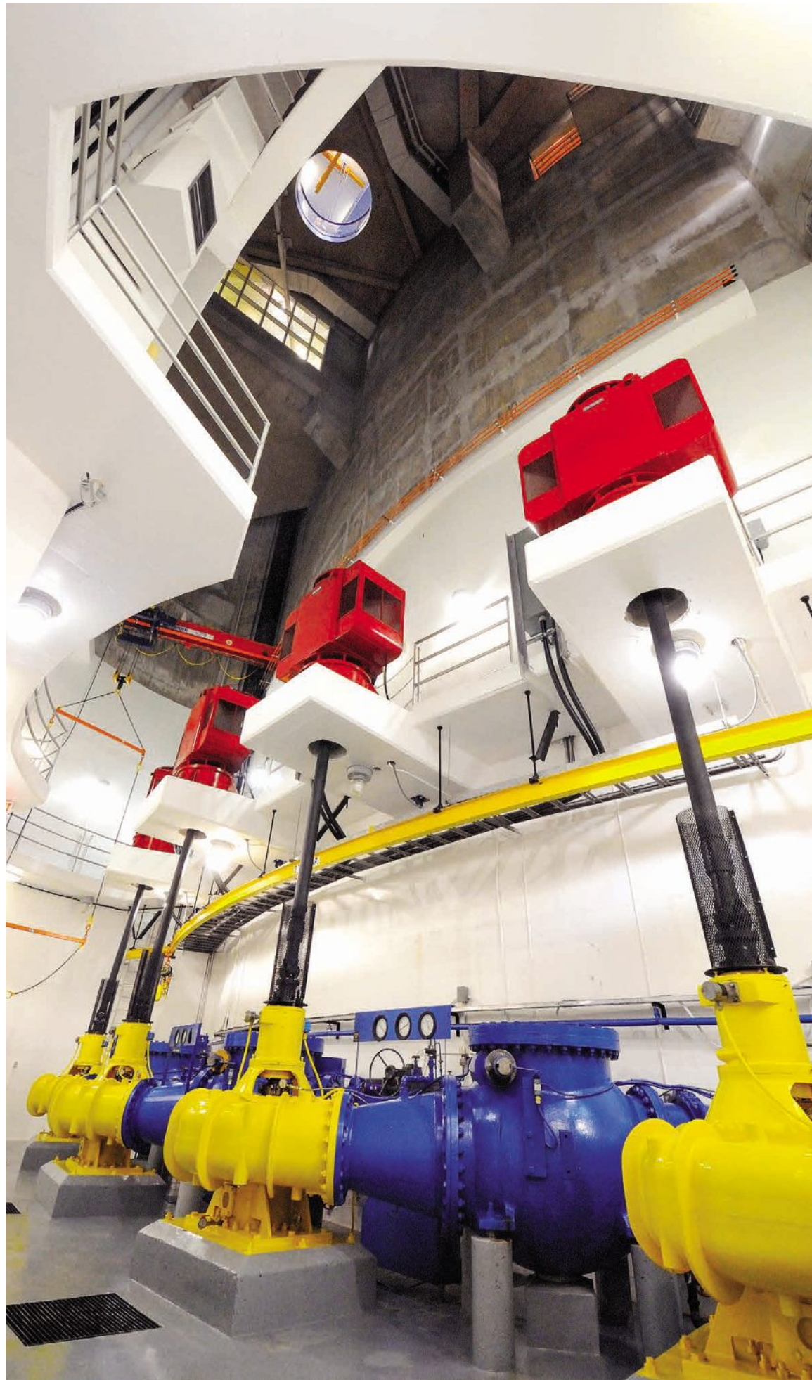
Inside the Riverview wastewater treatment facility.
