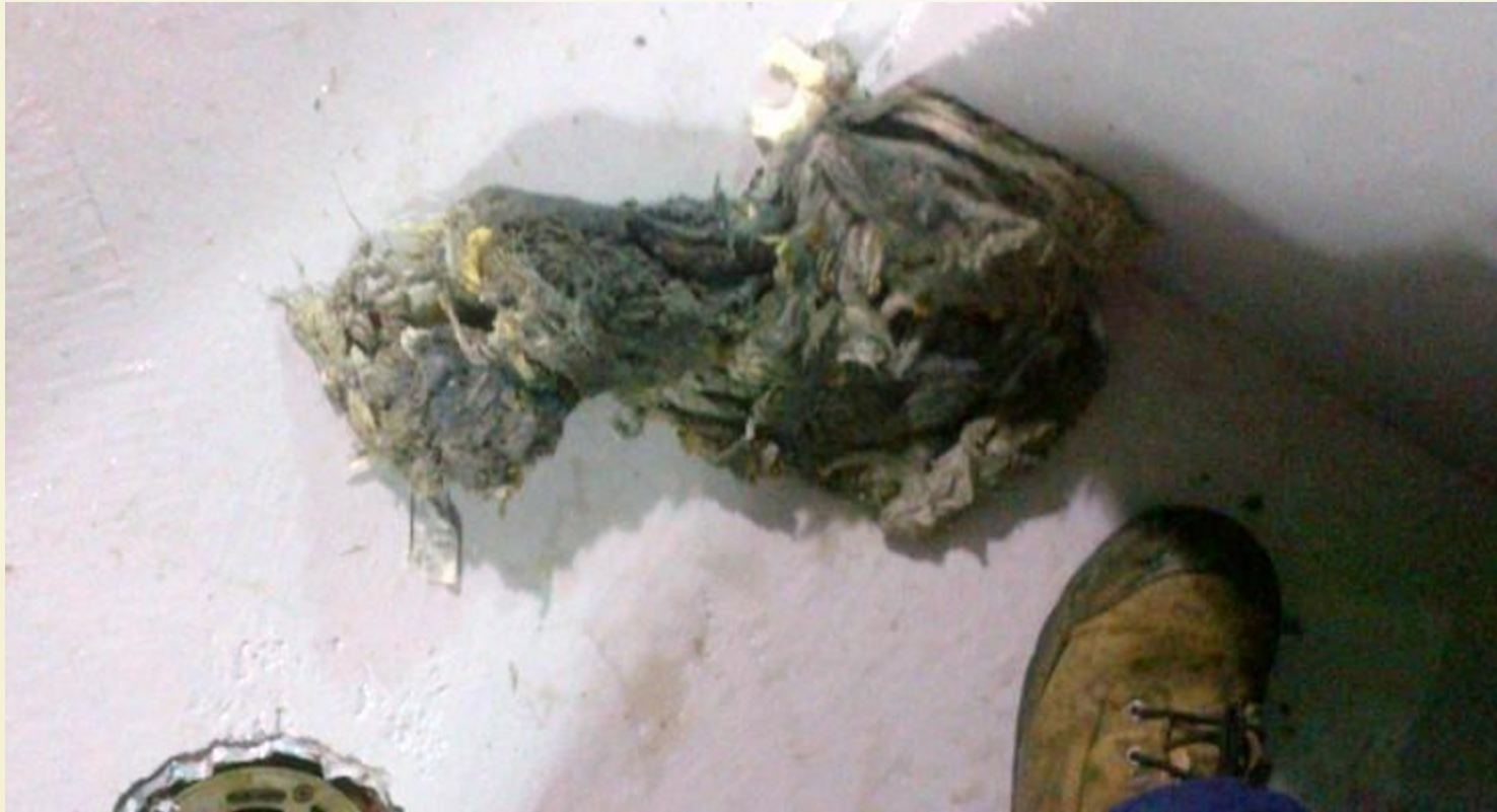
Material from plugged pump.
