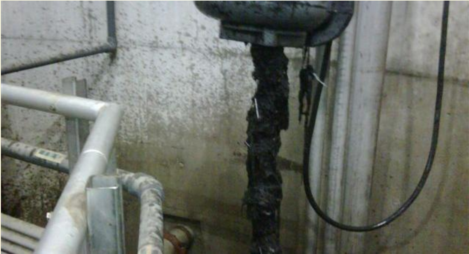
Plugged inlet to pump.
