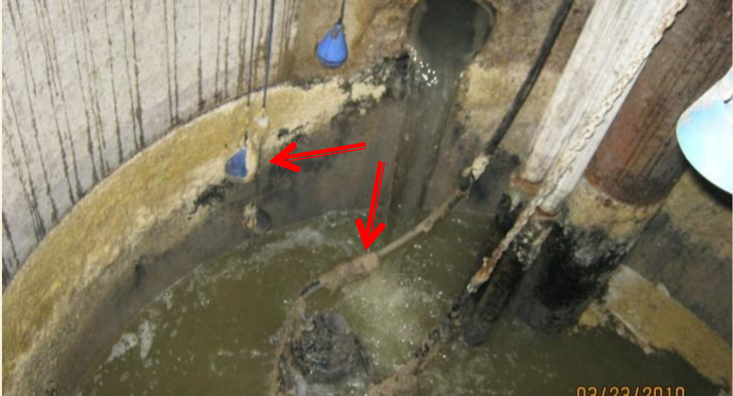
Pumping station ball floats and cable.
