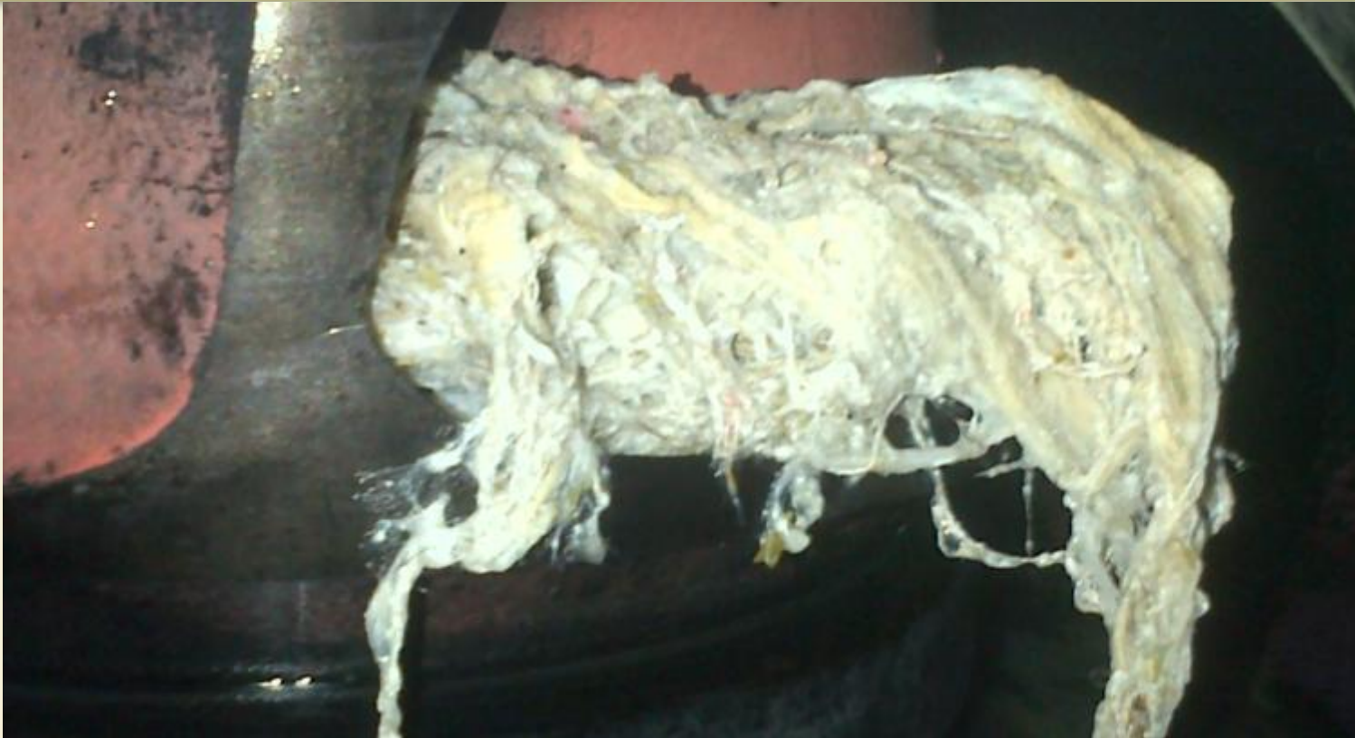
Pump impeller plugged.
