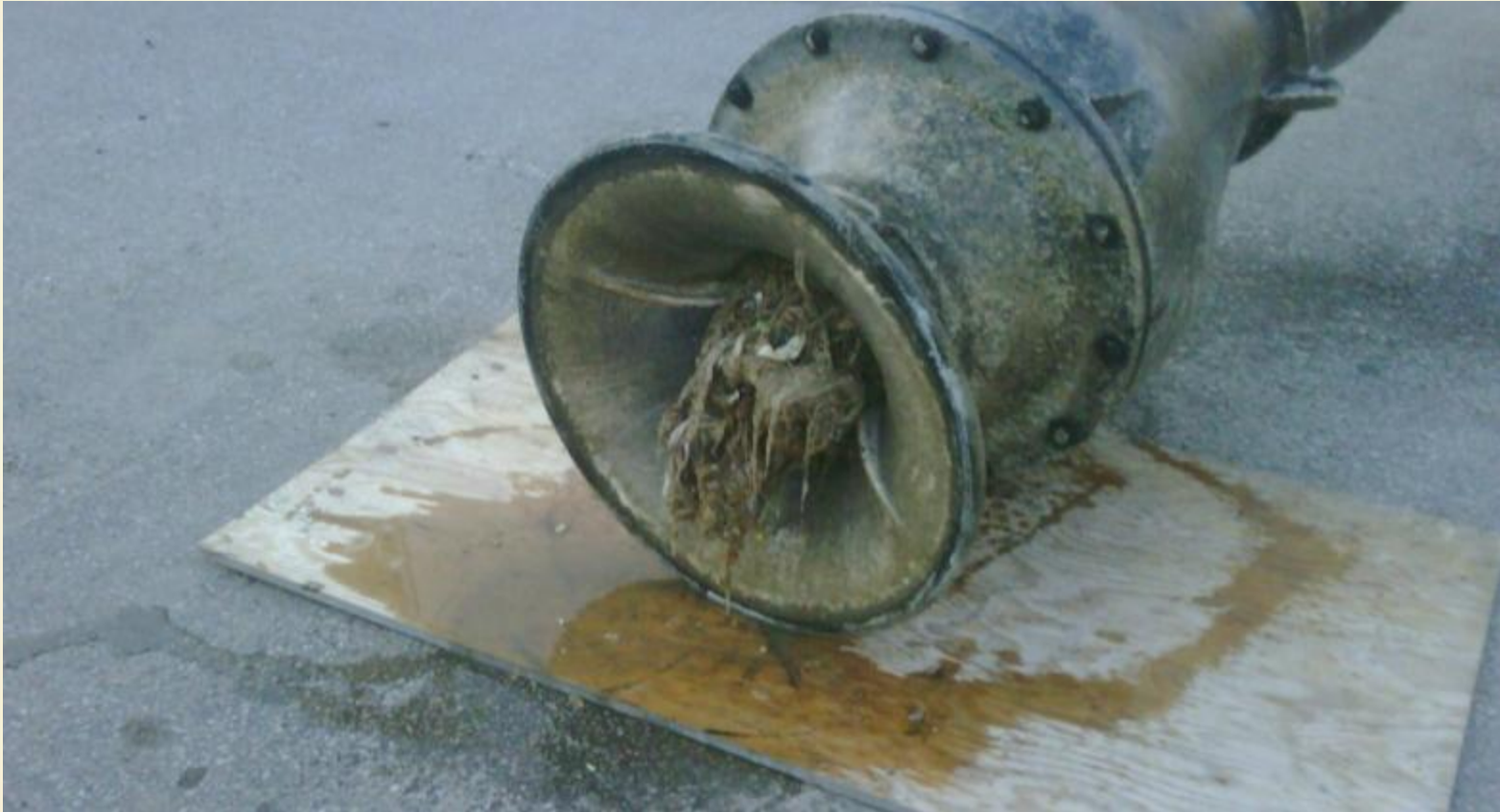
Inlet to pump.(Crane used to remove pump)
